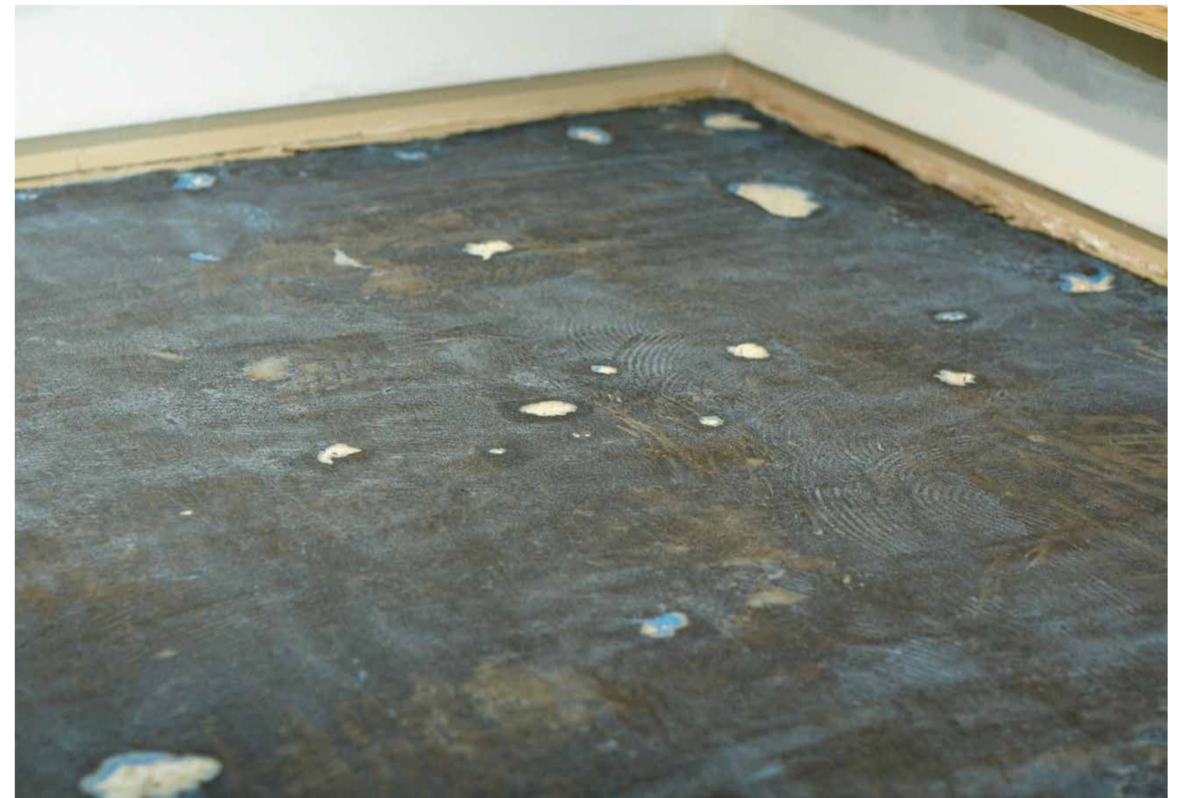
The depth of the dents and imperfections in the substrate can be seen more clearly just after the primer has been applied.
