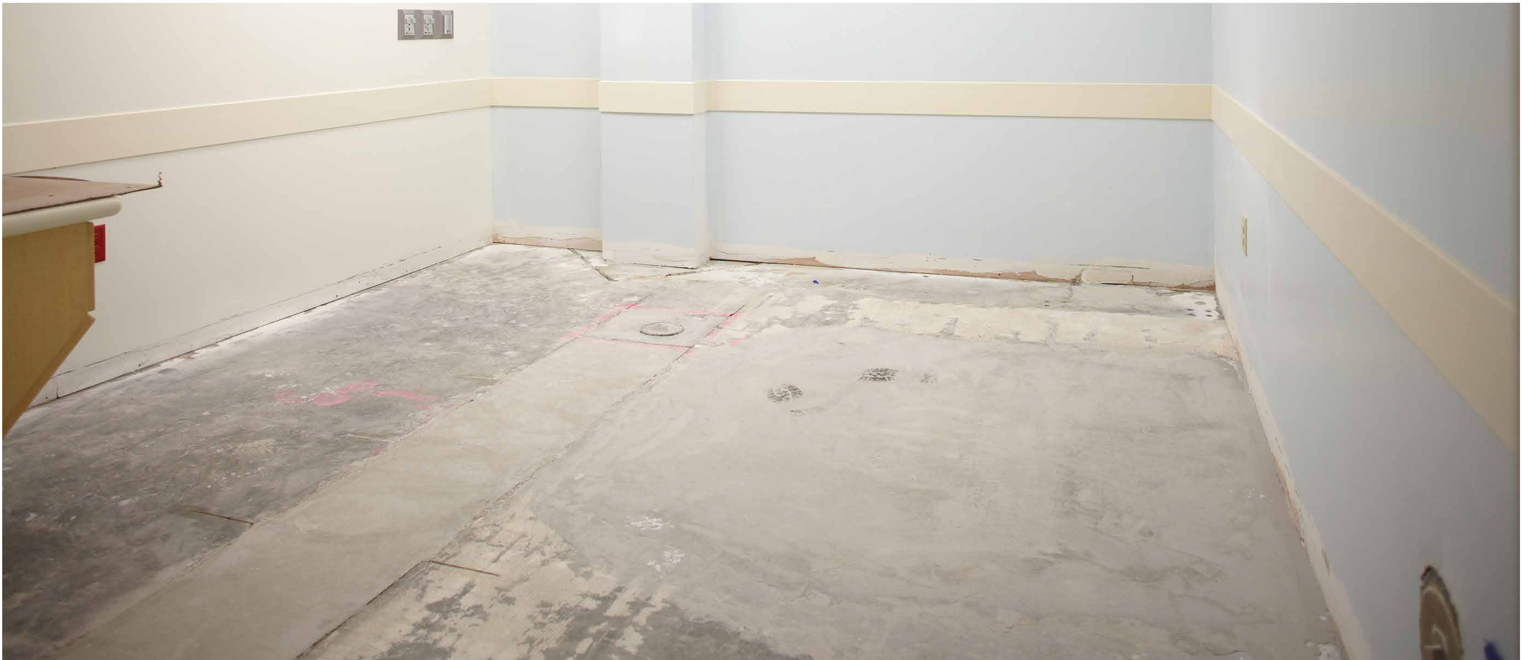
The existing concrete was uneven and in need of repair and leveling.
